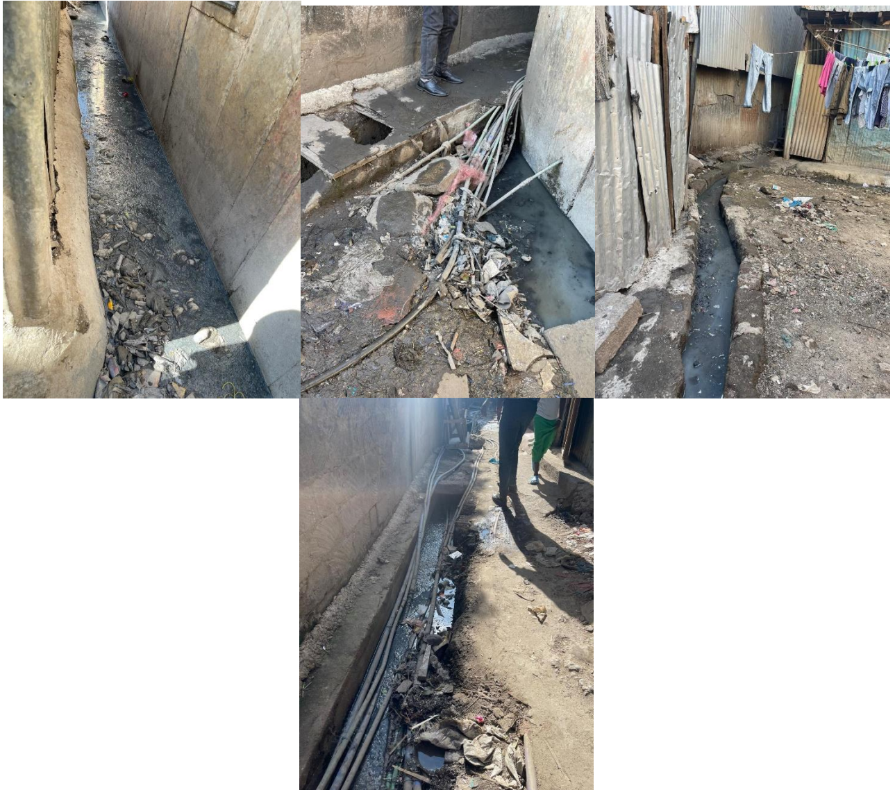
Figure 1,2,3,4: Above are sections of the Drainage system in Mukuru Kayaba that needs to be repaired, cleaned and de-silted.
