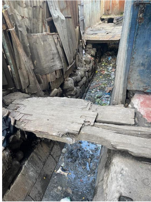
Figure 6: A section of a clogged drain along Tetra Pak Village Road
